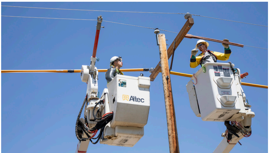
Co-op employees were given the chance to work on lines while the instructors offered tips during the field day portion of the Tech School. | PHOTO BY RYAN HALL
